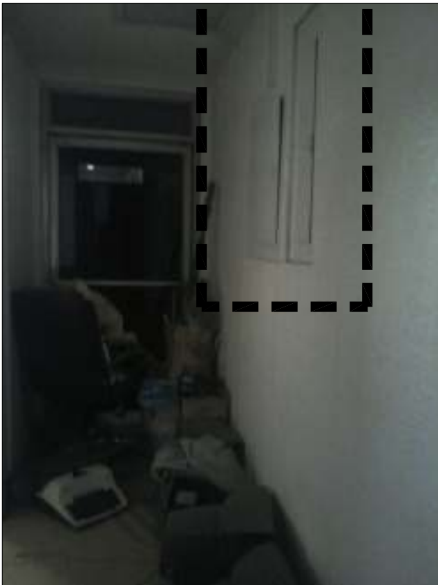
PROPOSED LOCATION OF NEW ATS BESIDE EXISTING ELECTRICAL PANELBOARD
